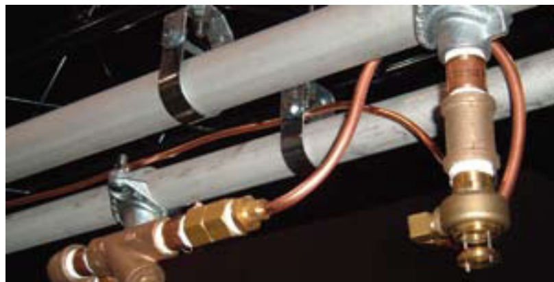
Emitter and Piping
